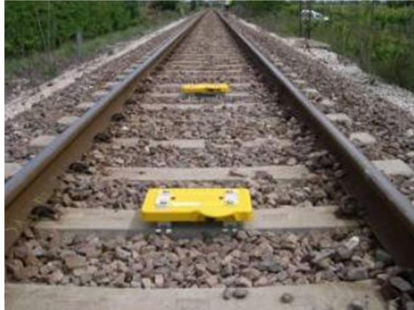
Figure 24: Eurobalises on a railway track
