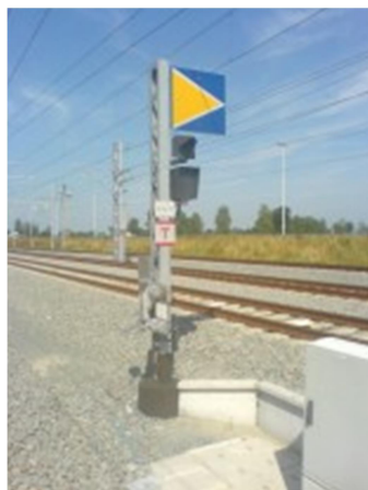
Figure 25: ERTMS/ETCS Marker boards
